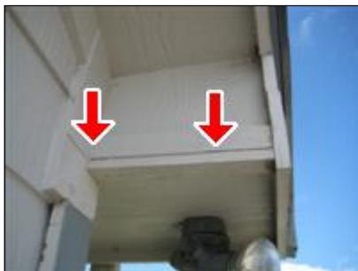
E. Picture 1 OPENINGS IN SOFFIT
