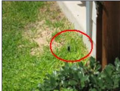
A. Picture 1 Zone# 3 damaged head
