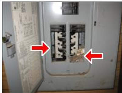
A. Picture 2 SUB-PANEL IN STABLES
