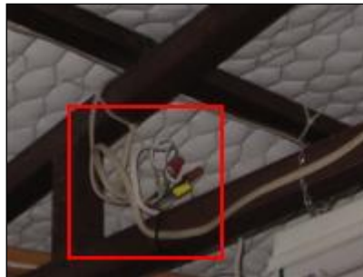
B. Picture 16 Missing J-Boxes at Metal Garage Lighting
