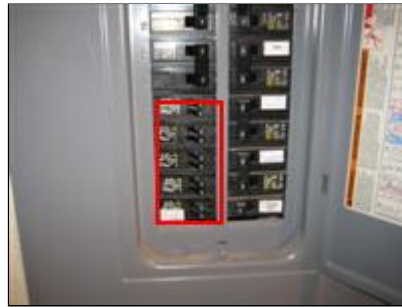
B. Picture 22 Missing AFCI Breakers
