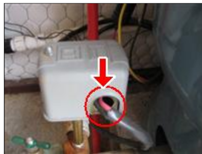
B. Picture 13 No wire stop at well pump
