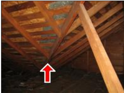
D. Picture 3 VALLEY RAFTER SUPPORT NEEDED
