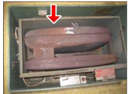
A. Picture 7 OLD & RUSTED OUT HEAT EXCHANGERS
