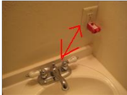
B. Picture 4 NO GFCI IN BATHROOMS
