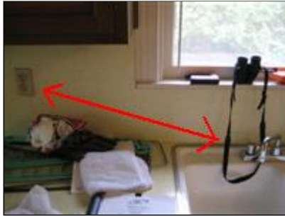
B. Picture 2 NO GFCI WITHIN 3' OF WATER SOURCE
