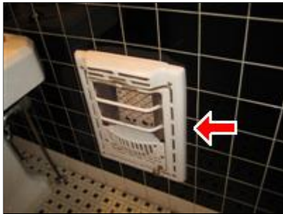
A. Picture 1 GAS WALL HEATER
