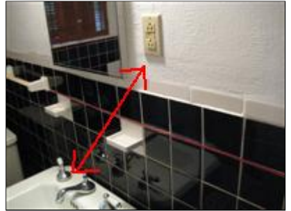
B. Picture 3 GFCI NON-FUNCTIONING
