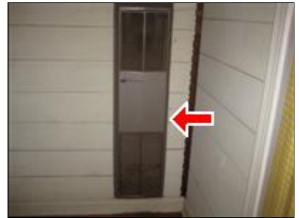
A. Picture 3 NO GAS TO WALL HEATERS
