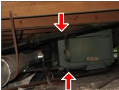
A. Picture 5 FLOOR FURNACE
