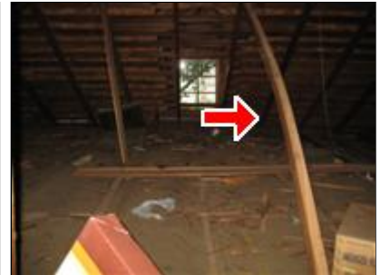
D. Picture 5 WEAK / UNSTABLE SUPPORTS
